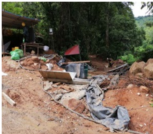
Poor housekeeping at the worksite in section-d, 5 Nov.2021
