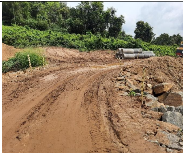
Stream blocking at access to T1 inlet portal Lel oya (22 Dec. 2020)
