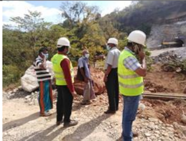
Joint site inspection with farmers to shift the irrigation canal at Lel oya 13 Oct. 2020
