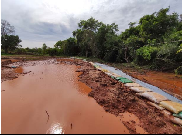
Overtopped sand bag barrier and siltation in tank
