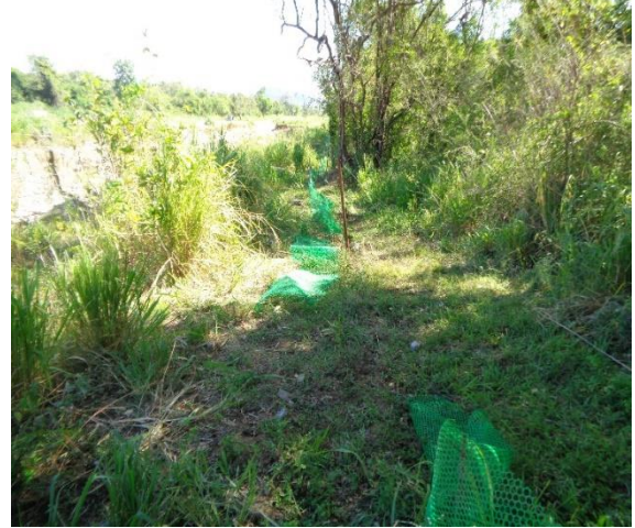
Collapsed safety net at section 2 (Since March 2020)
