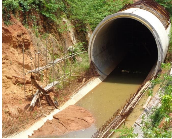
Collapsed canal banks in section 3 (May 2020)
