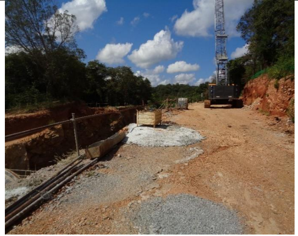
Concrete wastes are left in the site (Since March 2020)
