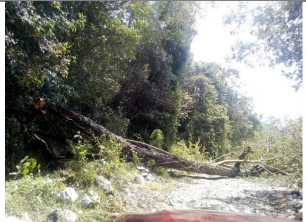
Clearing trees fallen to access roads to Tunnel 2 Outlet area in KMTC
