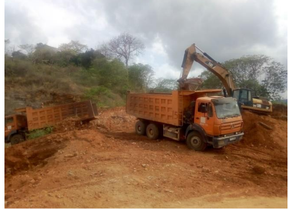
Access road preparation to facilitate the timber removal process by STC in KMTC open canal area
