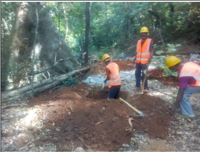
Land preparation for root ball tree planting at 168m (LM 9) on LHS
